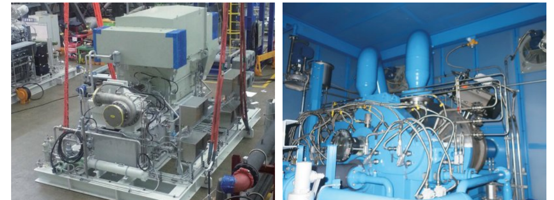
MENA Power Plant FGC
